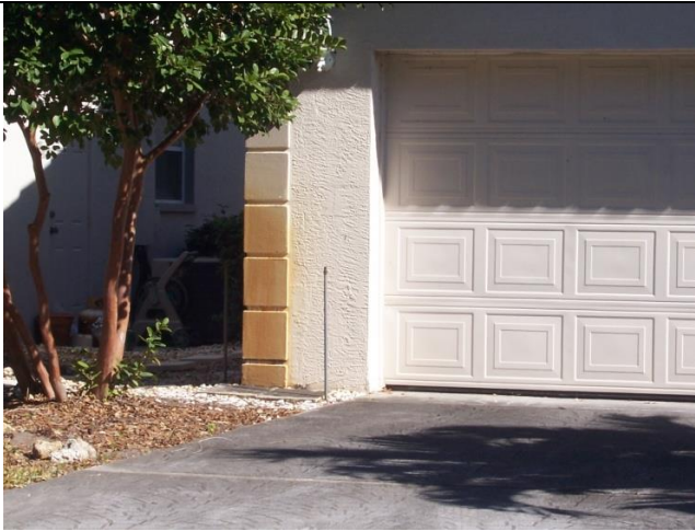
Stains from irrigation system
