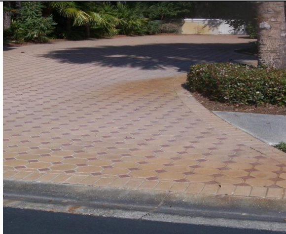
Sprinkler water stains
