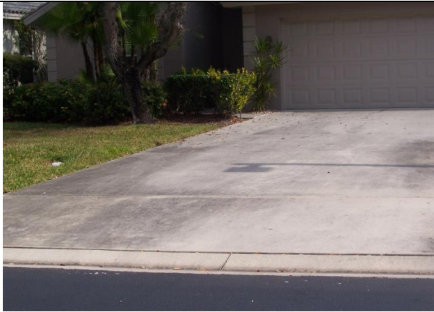
Dirt / Mildew stained concrete
