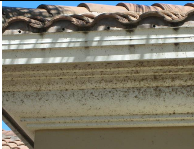
Fascia dirty - needs painting or pressure washing
